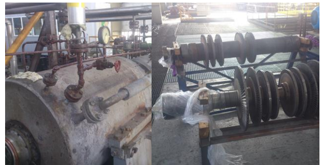
Fig. 10. Turbo generator and high and low decompression stage rotors
